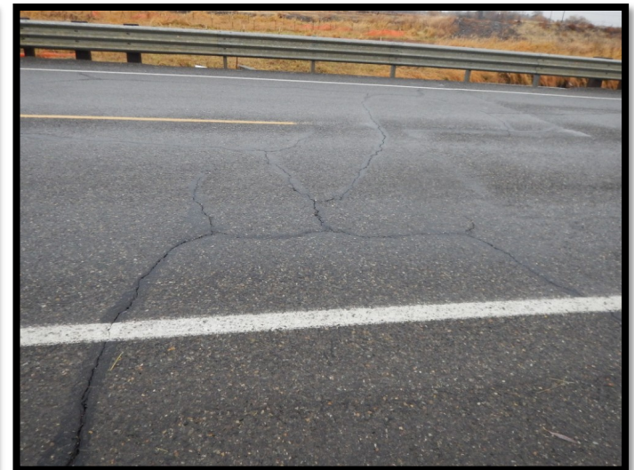
Cracks in bridge surface
